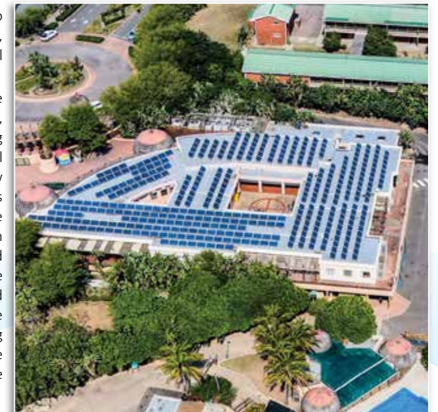
Solar panels on the roof of the SAAMBR administration offices.
